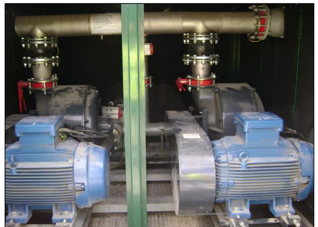
Duty – Standby Belt Drive blowers
