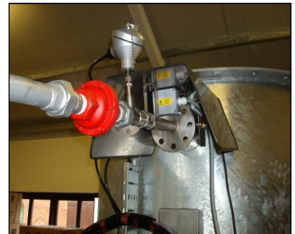
Fireblaster landfill gas Pilot
